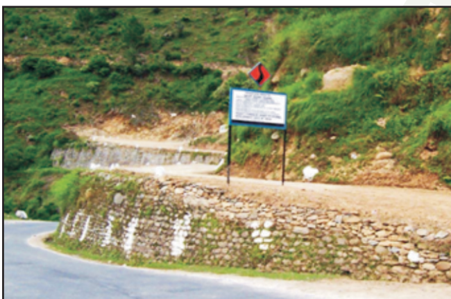
Photograph 5 - Improper Sight Distance- A Safety Hazardous Condition at PMGSY Roads
