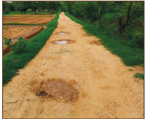
Figure 4: Potholes on gravel road
