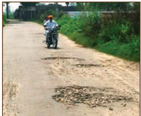
Figure 5: Potholes on a paved road
