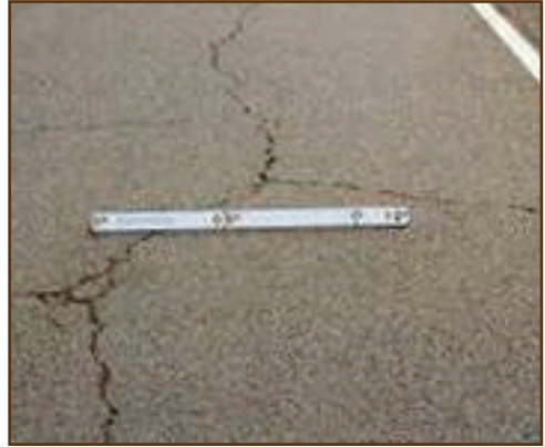
Figure 9: Cracks on pavement
